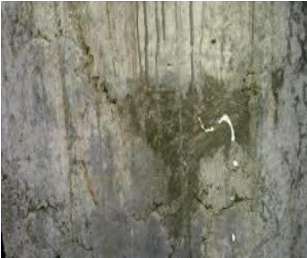
Fig -3 Seepage due to cracks
