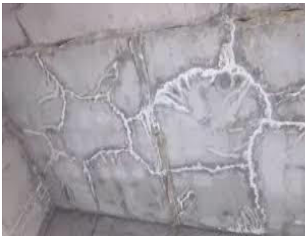
Fig -4 Leakage in Slab
