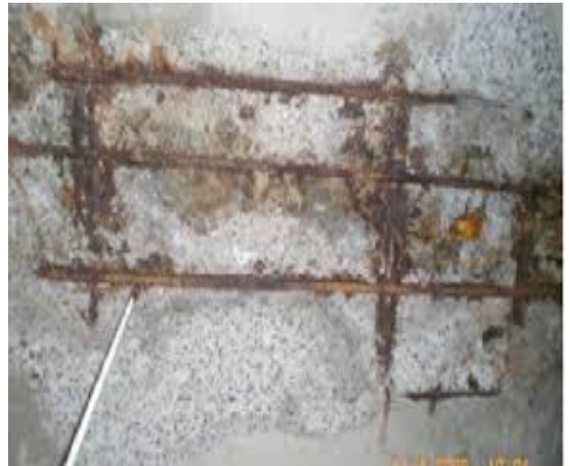
Fig -1 Slab Reinforcement Corrosion
