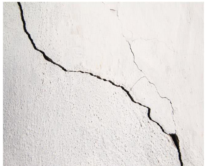
Fig -2 Plaster cracks on external wall
