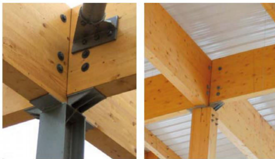
Fig.6.14 Head of the wood segment (left) and steel section (right) to glulam rooftop part
