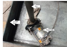
Fig No. 3.4. Water Pump
