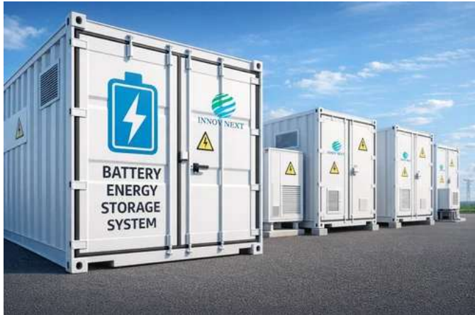
Fig 2- Battery Energy Storage System
