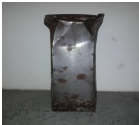
Fig 12: Failure of welded column
