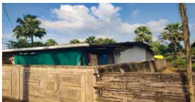
Figure 6. External wall and boundary masonry at a second surveyed property, showing weathering and surface staining consistent with prolonged moisture exposure.
