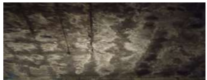
Figure 1. Close-up of an RCC slab soffit showing extensive moisture staining, efflorescence, and surface deterioration consistent with long-term water ingress through an unwaterproofed terrace.
