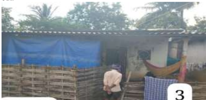
Figure 3. Temporary tarpaulin sheeting deployed over a damaged roof section by a beneficiary household as an interim measure against active slab leakage.
