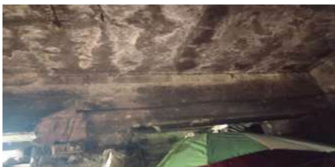
Figure 2. Interior room corner showing heavy fungal staining at the slab-wall junction and degraded surface-mounted electrical wiring routed through the damp zone — a combined structural and fire-safety hazard.
