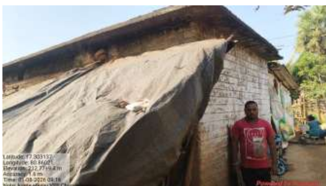
Figure 4. Tarpaulin-covered roof at a second affected house, illustrating the prevalence of this informal coping measure across the surveyed cluster prior to rehabilitation.
