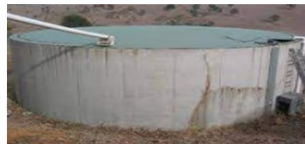
Fig. 3 Partially Underground Water Tank
