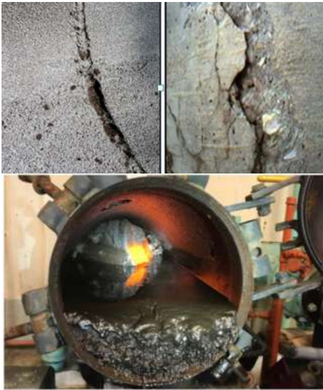
Figure 1. Internal pipe leakage and choke
