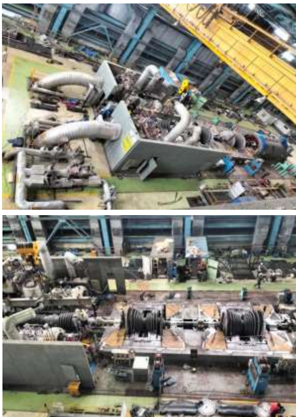
Fig.3.Steam Turbine Alignment Monitoring System at Thermal Power Plant Koradi
