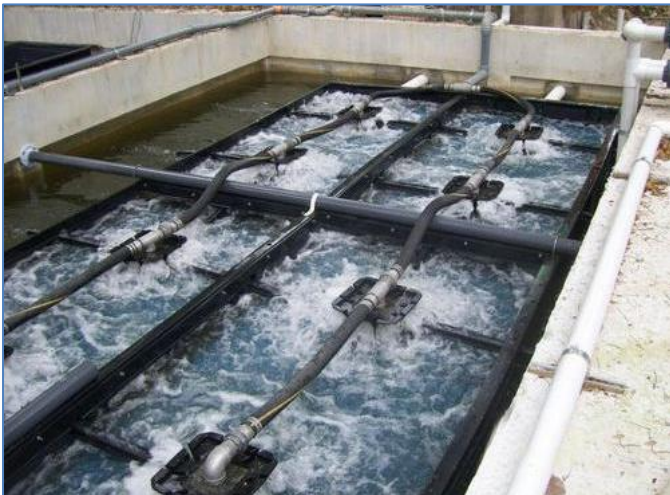
Fig -4: Aeration Tank at current WWTP at Okhla District
