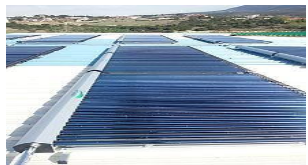
Fig. 3.2 Evacuated Tube Collector
