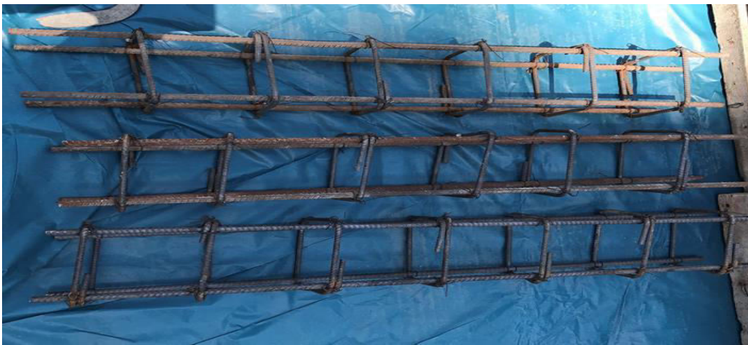
Fig No. 2 square shape stirrups reinforcement
