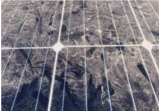
Figure(4) Dust accumulation on solar panel.
