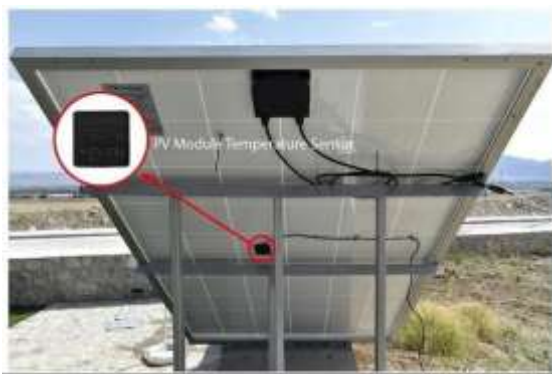
Figure(3) Thermal monitoring system.
