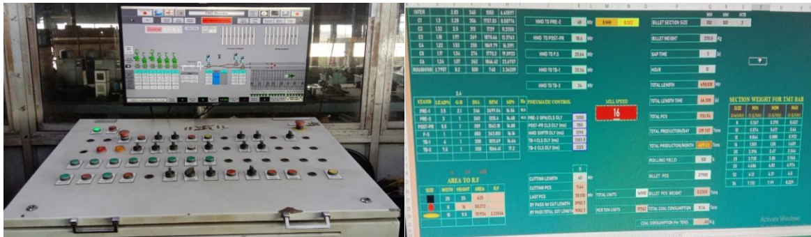
PLC VEGA CONTROL SYSTEM
