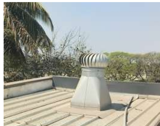
FIG 9- AIR DUCTS AT STUDIO 888 IN SANGLI
