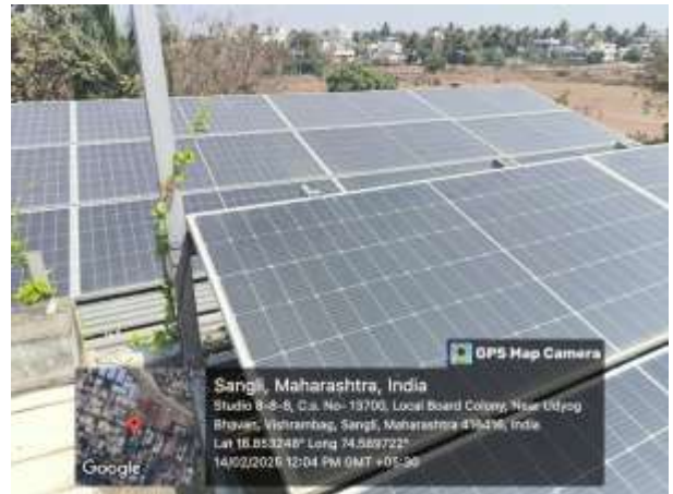
FIG 3- SOLAR PANEL AT STUDIO 888 IN SANGLI
