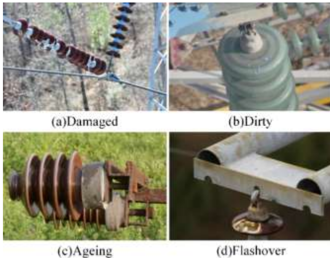
Fig.1: Several common insulator defects.
