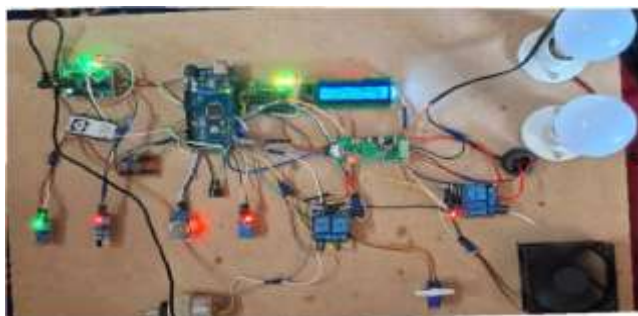
Fig.4 System Tripped Due to OverLoading
