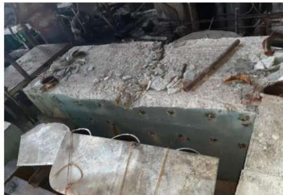
Figure 3: Spalling and crushing of top chemical grout of Pedestal B4
