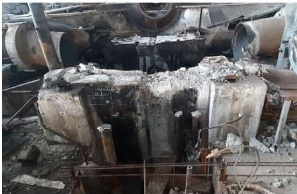
Figure 2: fire-damaged face of Pedestal B2
