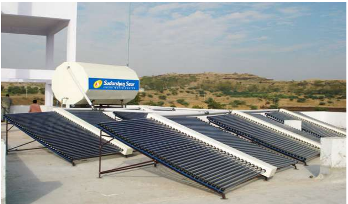
Fig: 3.3 Solar Arrays of capacity 500 Liters each
