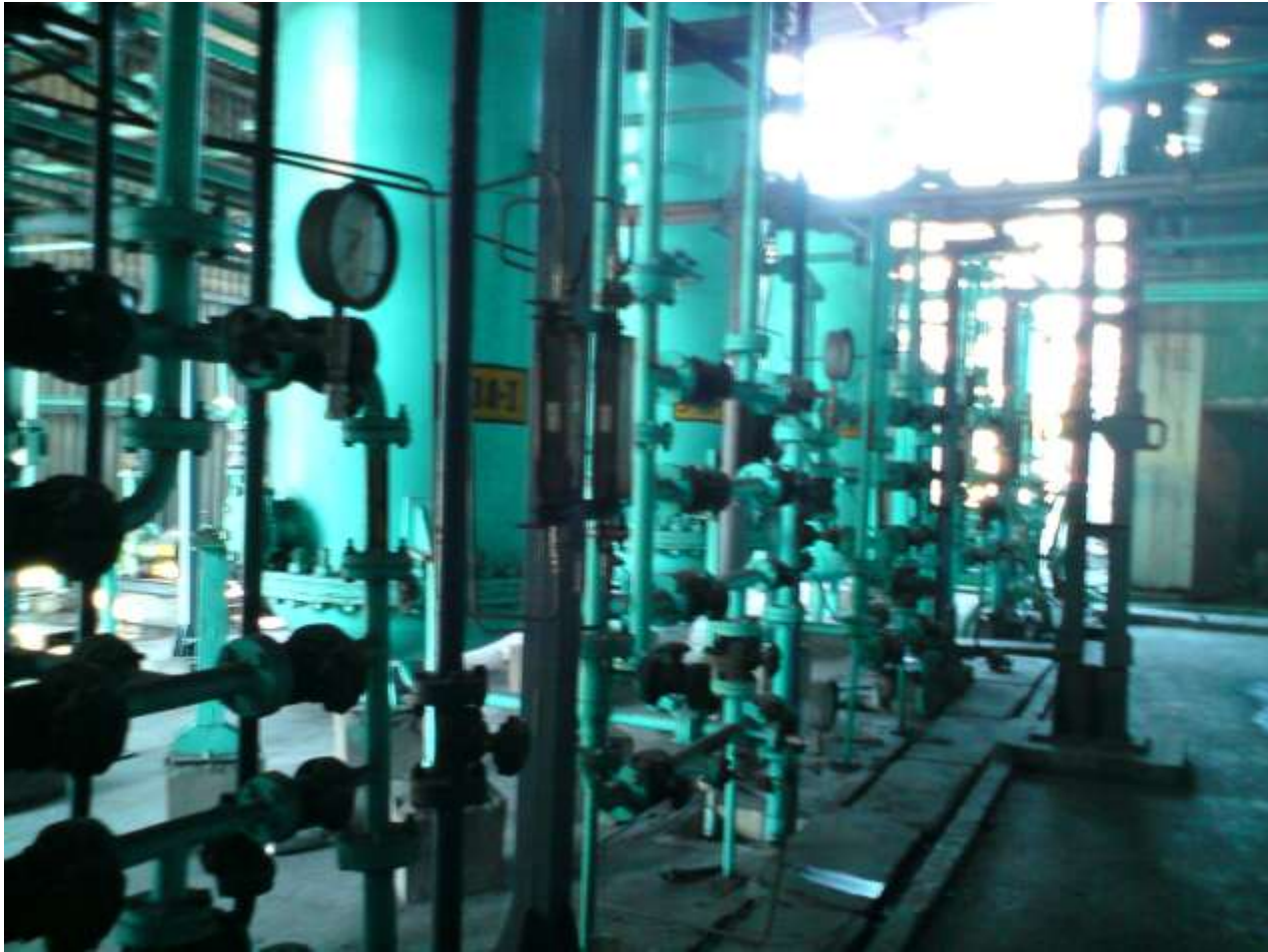
Fig: 3.6 Water treatment plant of 64 MW Thermal power Plant
