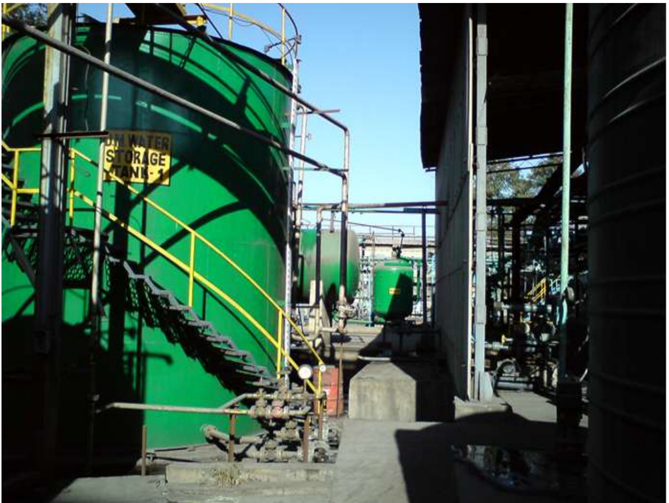
Fig: 3.8 DM Water Storage tank-2 of capacity 100KL
